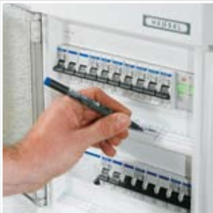
Large area for labelling - and a lot of space to actuate the equipment installed.
