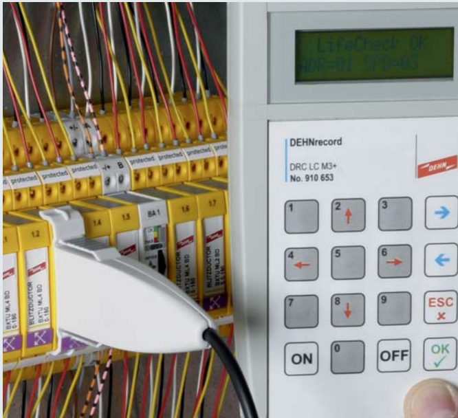
Testing of an SPD module via RFID technology (LifeCheck)
