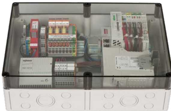
The compact WAGO telecontrol solution with DEHN arresters is installed in transformer substations.
