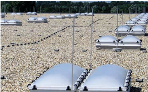
Figure 5.1.1.19 Flat roof with air-termination rods and conductor holders: Protection of the domelights
