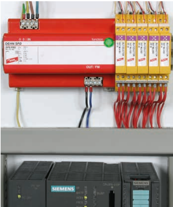
Figure 7.7.3.1 Protection of industrial electronic equipment (e.g. a PLC) by BLITZDUCTOR XT and SPS Protector
