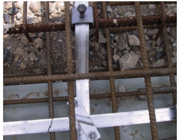
Figure 5.5.2.4 Foundation earth electrode in use
