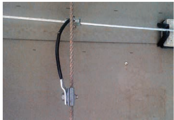
Figure 5.1.12.2 Incorrect installation: Safety rope system intersects the air-termination system
