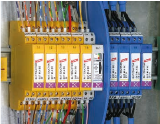
Figure 8.2.6.3 Monitoring of surge protective devices by means of the DRC MCM XT condition monitoring unit
