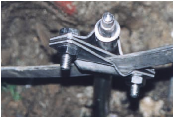
Figure 5.9.4 Connection of an earth rod to the ring earth electrode of the station
