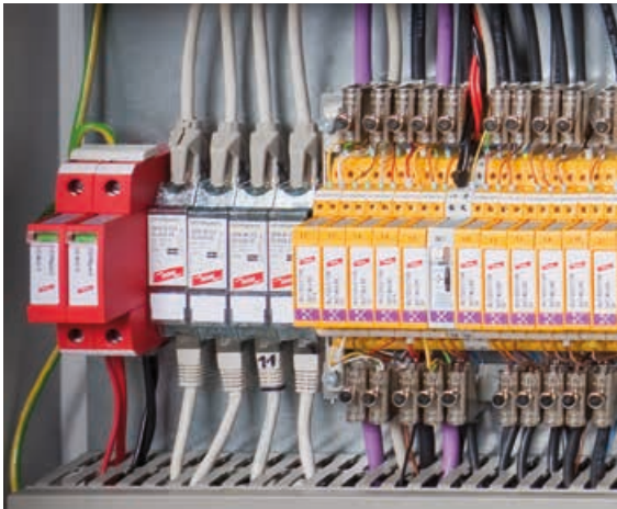
Figure 9.16.11 Example of surge protective devices in a pitch system
