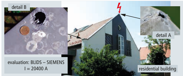
Figure 5.1.4.2 Example of damage: Sheet metal
