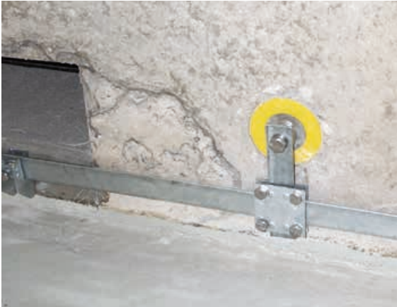
Figure 7.7.1.1 Ring equipotential bonding and fixed earthing terminal for the connection of metal installations
