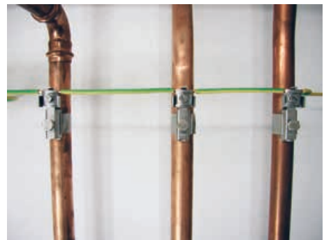
Figure 6.1.6 Through-wired equipotential bonding bar
