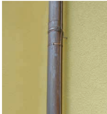
Figure 5.2.2.2.4 Down conductor installed along a downpipe
