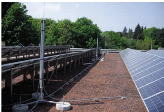
Figure 5.2.4.5 Protection of a PV system by means of a HVI light Conductor
