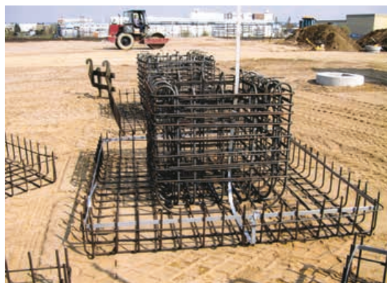
Figure 5.5.2.24 Foundation earth electrode for pad foundations with terminal lug; source: Wettingfeld, Krefeld
