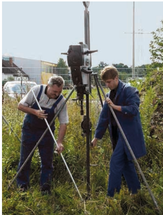
Figure 5.5.4.2 Driving an earth rod into the ground by means of a hammer frame and a vibration hammer
